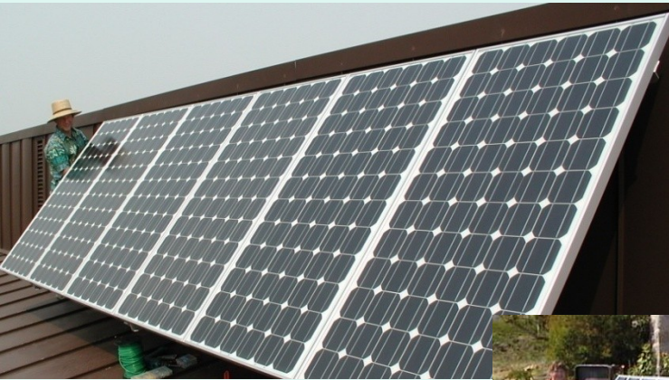
Photo: Lincoln Electric Co-op / Thirsty Lake Solar
