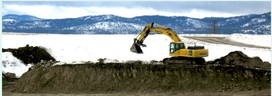
Flathead County Landfill Gas Project
