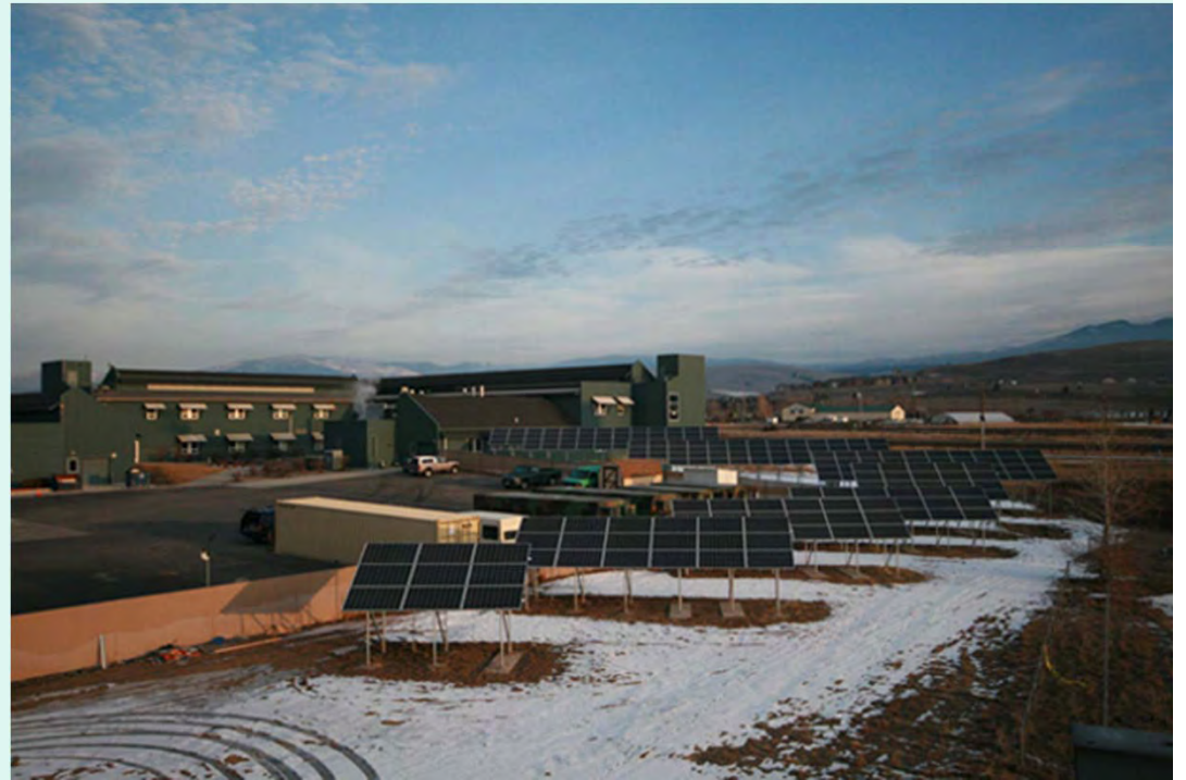
50 kW solar system in Missoula (Oasis Montana)
