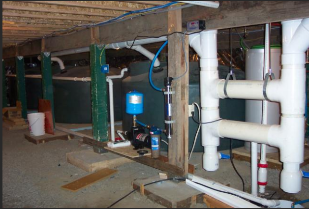
Crawlspace with collection tanks, booster pump, particulate and UV filters. Sediment catcher in foreground.
