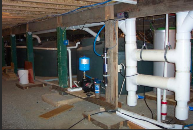
Crawlspace with collection tanks, booster pump, particulate and UV filters. Sediment catcher in foreground.
